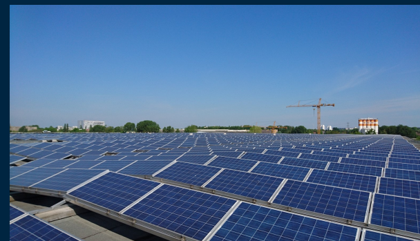
Photo of Solar PV in Berlin, roof mounted: divested
